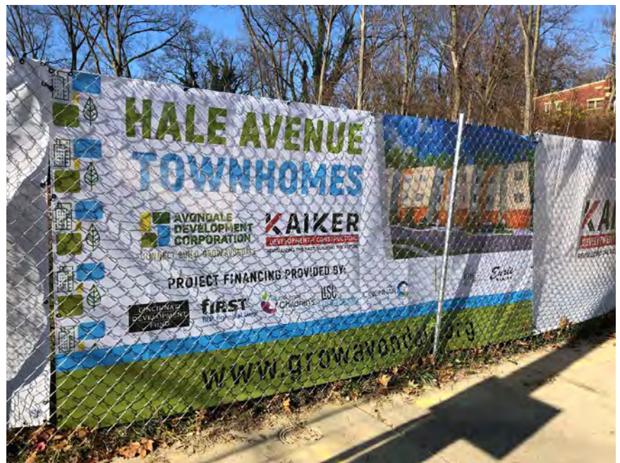
A project under construction funded through Cincinnati's CDFI, the Cincinnati Development Fund.
