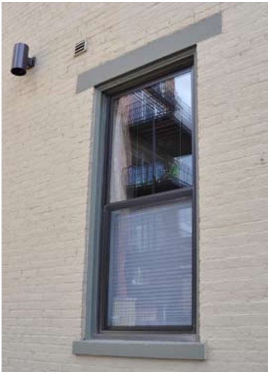
[ PHOTO 11 ] An example of an aluminum replacement window on a rear elevation of the building. Note how only the material is different; window still has the look of a wood window.
