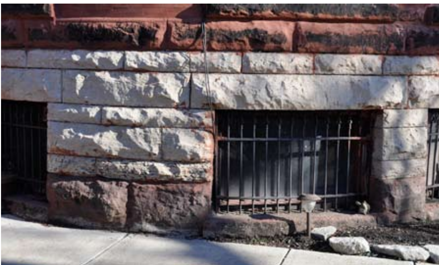
{PHOTO 2} Rock-faced sandstone blocks form a distinctive foundation on this 19th century home. Note the wrought iron security grille at the window opening.
