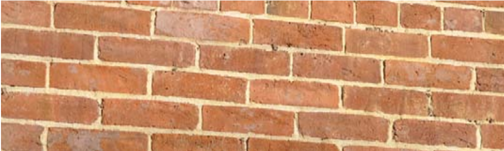
[ PHOTO 8 ] — In addition to matching the joint tooling, be sure that the mortar mix, texture and color is appropriate for the historic masonry.
