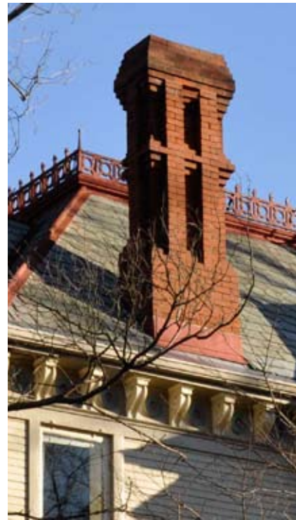
[ PHOTO 7 ] Corbelled chimney, iron cresting and ridge caps on a slate roof.
