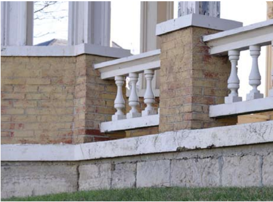
{ PHOTO 5 } — This porch foundation, with its distinctive stone water table, is an architecturally significant feature of the house and should be maintained along with the main building foundation.
