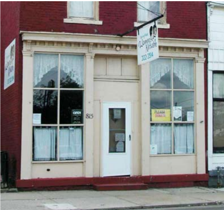
[ PHOTO 1 ] Although the entrance has been filled in with a smaller door, this is a good example of a 19th century storefront in Springfield. Instead of a transom, the display windows to either side of the door are tall.
