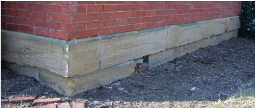
{PHOTO 1} A foundation of cut sandstone blocks that form a water table for this brick building.
