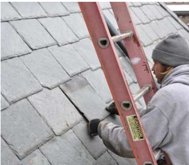
[ PHOTO 4 ] A workman replaces an individual damaged slate with a new slate that has been carefully selected to match the size, color and qualities of the original.
