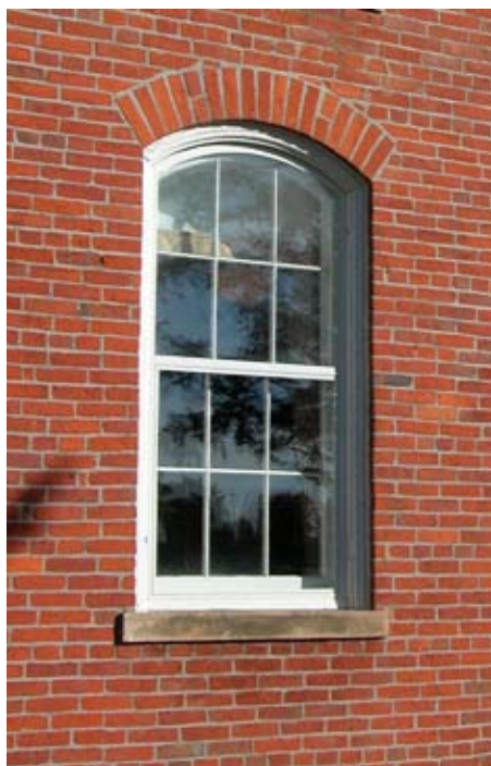
[ PHOTO 10 ] An example of a wood window replacement that matches the historic window exactly, including material.
