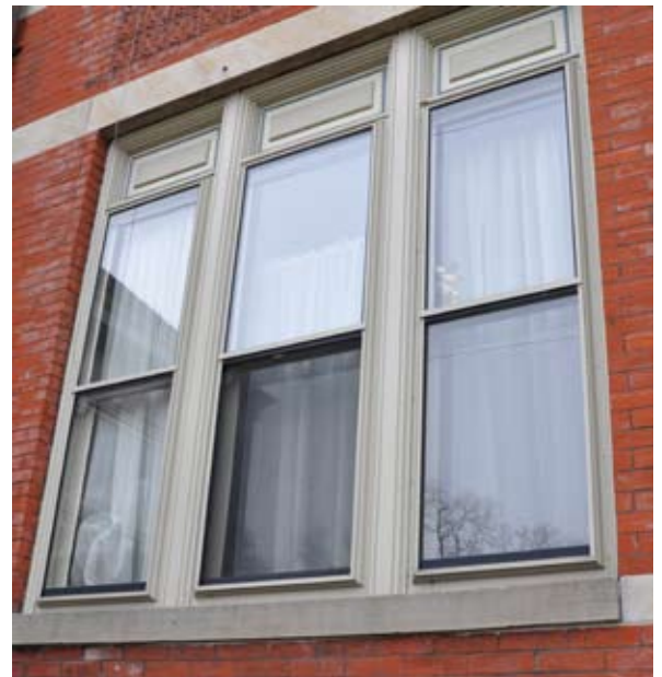
[ PHOTO 12 ] These storm windows fit the openings exactly, match the trim color, and provide insulating protection for the historic wood windows.
