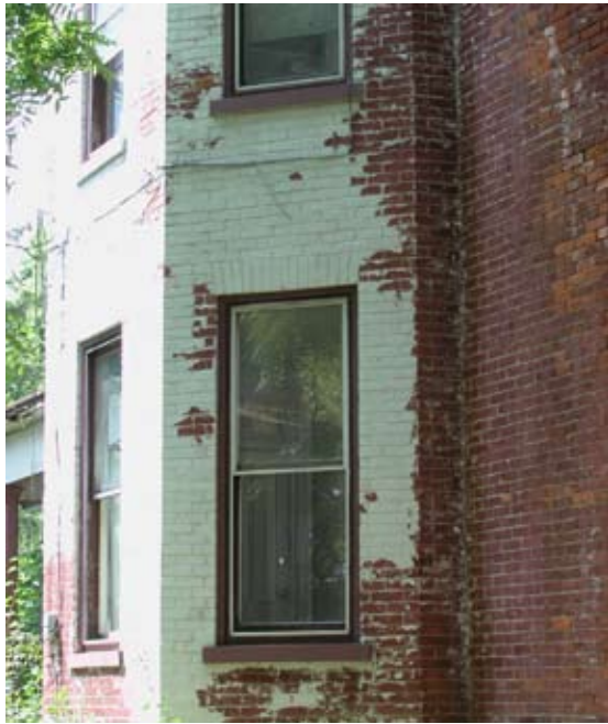
[ PHOTO 10 ] Paint removal from brick or stone can be difficult to achieve and is not always recommended. It must be carefully done to ensure that the masonry itself is not damaged.
