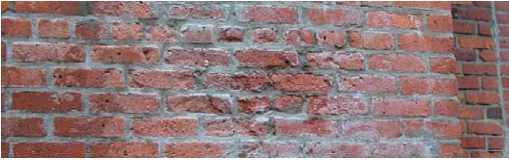
{ PHOTO 6 } Damage to the masonry is evident on this wall, which has suffered from poor repointing techniques and moisture penetration that caused efflorescence and spalled brick.
