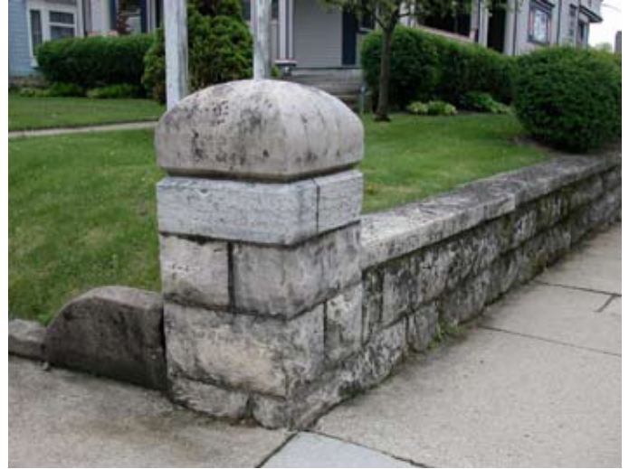
[ PHOTO 4 ] A limestone pier marks the corner of this property, with the retaining wall lining the property beyond.
