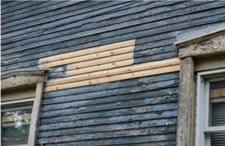
{PHOTO 12} An example of damaged siding that has been replaced with individual boards to match the existing.
