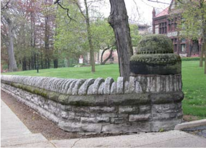
[ PHOTO 3 ] A distinctive stone retaining wall borders the Bushnell property on East High Street.
