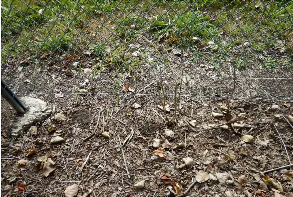
Photograph 25. Photo showing base of the 10-ft perimeter fence resting at or slightly above grade. Area 11 on Figure 4, view to the south behind Small Wooded Lot 4 along the southern boundary of SGH.
